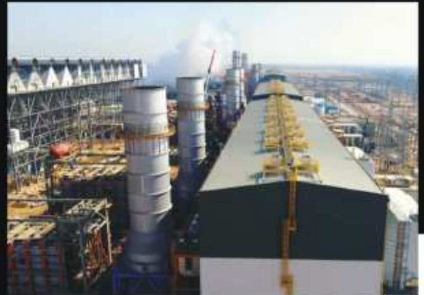
BESMAYA (BAGHDAD) GAS POWER STATION
